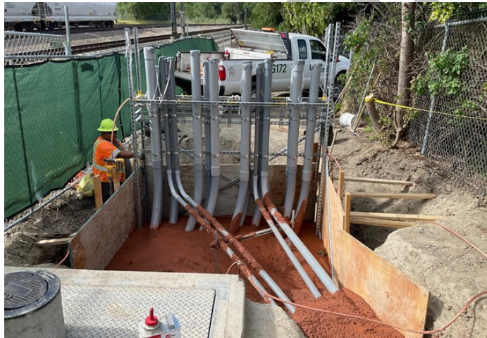
New UTA Disconnect Switch Ductbank
