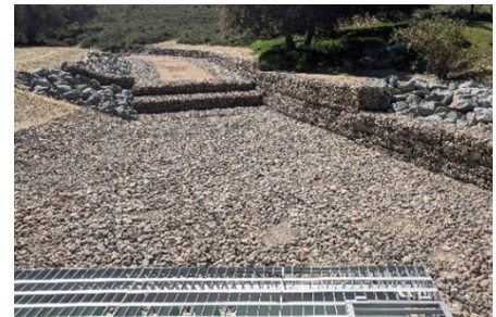
Balancing the design need for a large stormwater conveyance system to alleviate flooding with aesthetics.
