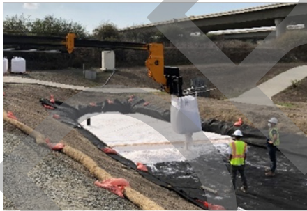
WSP provided on-site construction oversight of the Austin Sand Filter retrofit to ensure that the treatment BMP was installed per plan.
