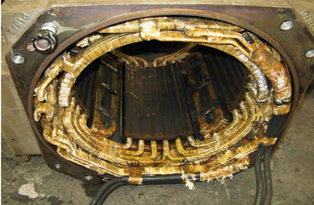
Figure 3 - Motor cleaned with improper chemicals
