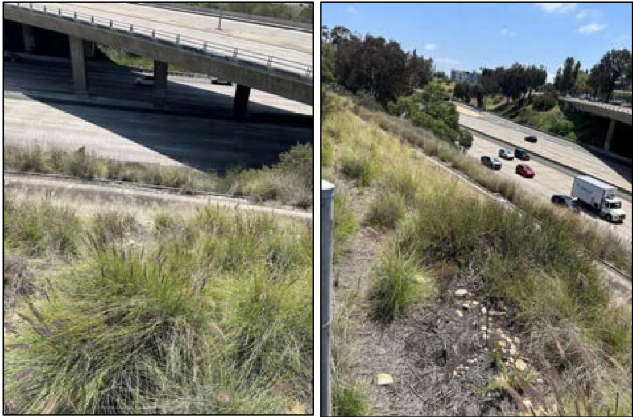
Figure 2-10 Caltrans Drainage Swale at Top of Slope
