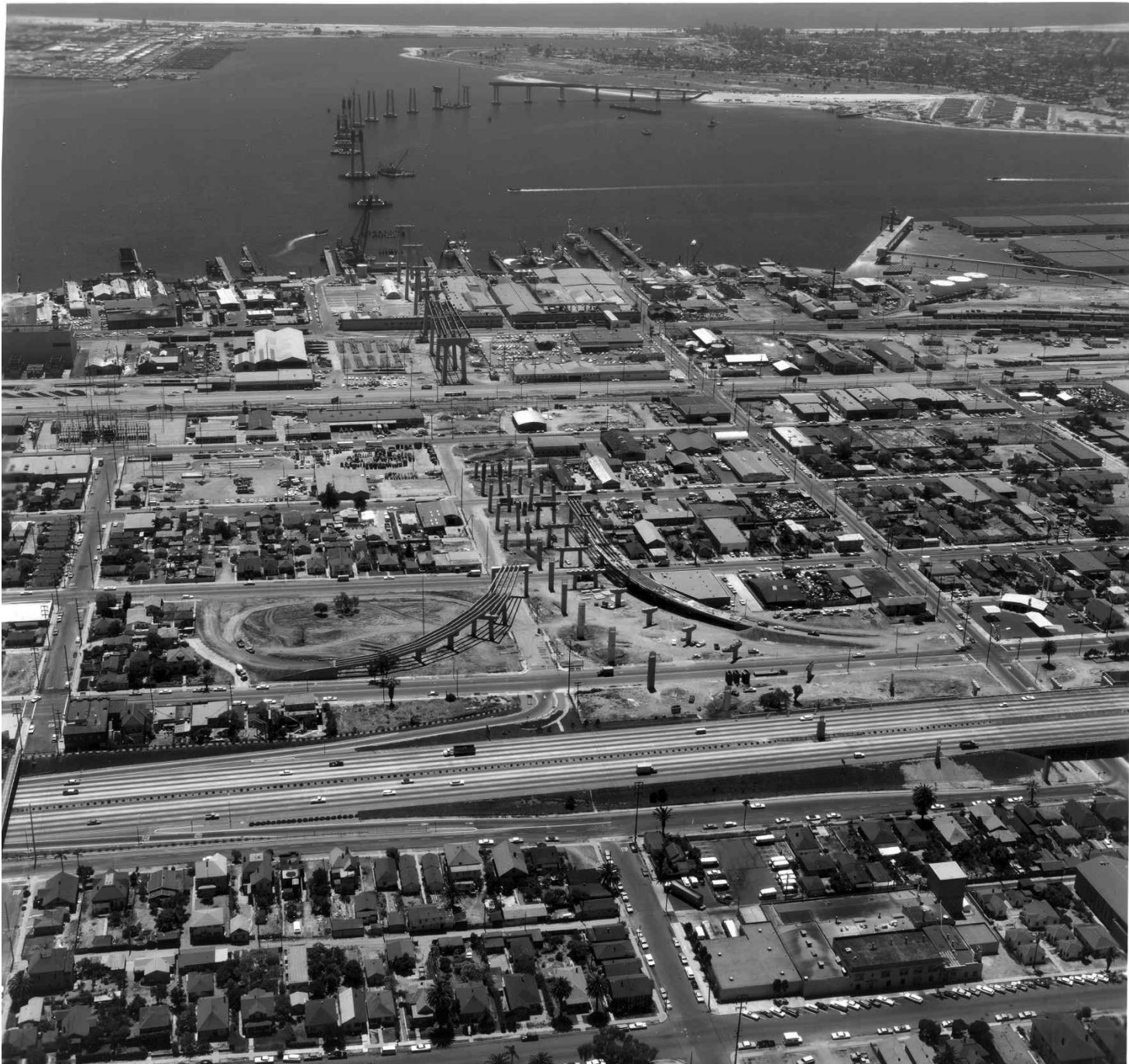
Primary Source 21 – The photo was shot looking west to show progress on the construction of the 11,179-foot-long concrete/steel girder San Diego-Coronado Bridge. The bridge opened August 3, 1969, replacing ferry service that had operated between San Diego and Coronado since 1886. 1967 photo courtesy of Caltrans.
